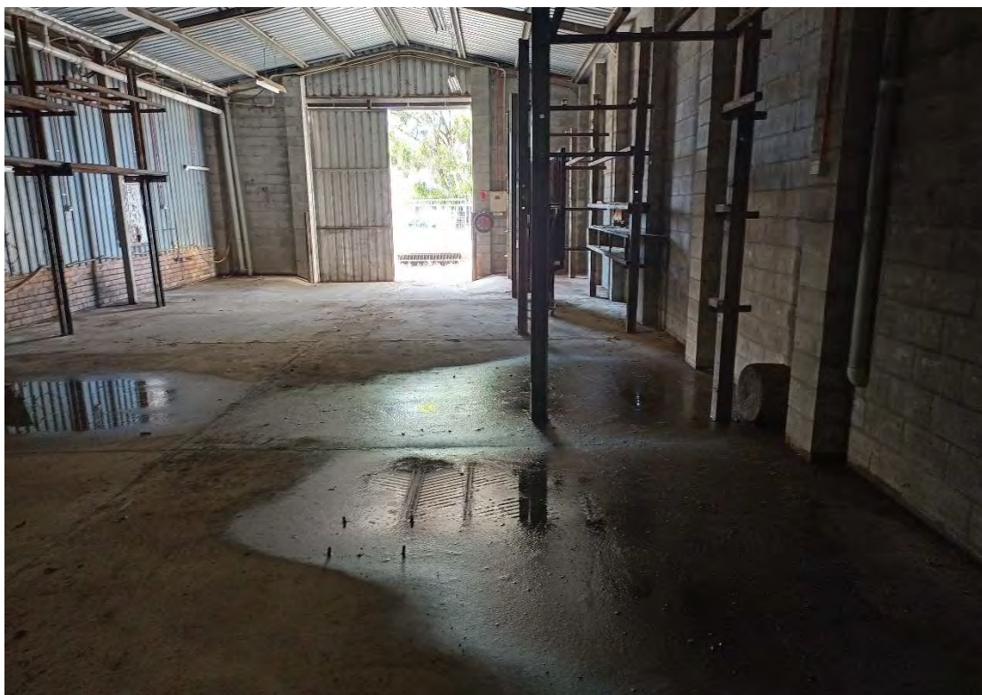
Photo 11: Shed in south eastern corner of the site. Hydrocarbon staining observed at surface (18 April 2024)
