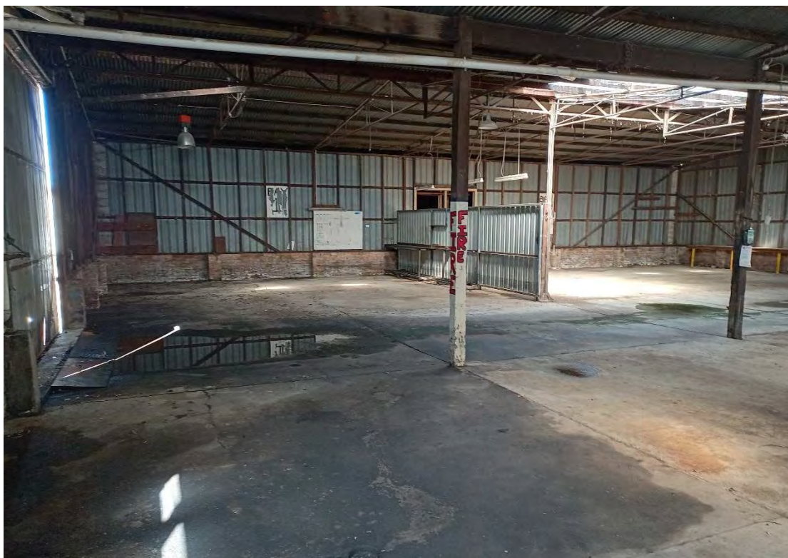
Photo 5: Former workshop area in eastern portion of the site. Hydrocarbon staining observed at surface
