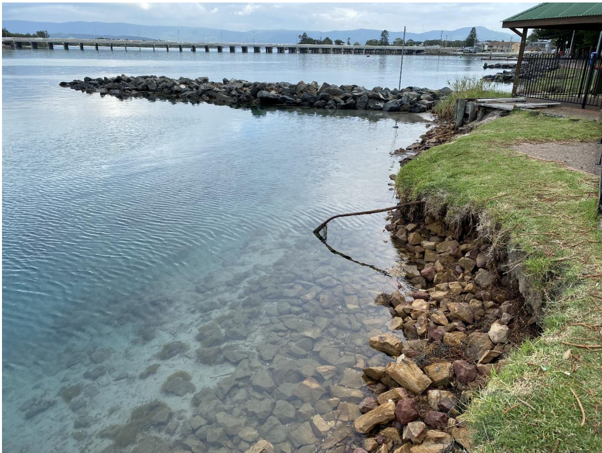
Figure 2.1 Erosion along the Windang foreshore immediately downstream of the groyne
