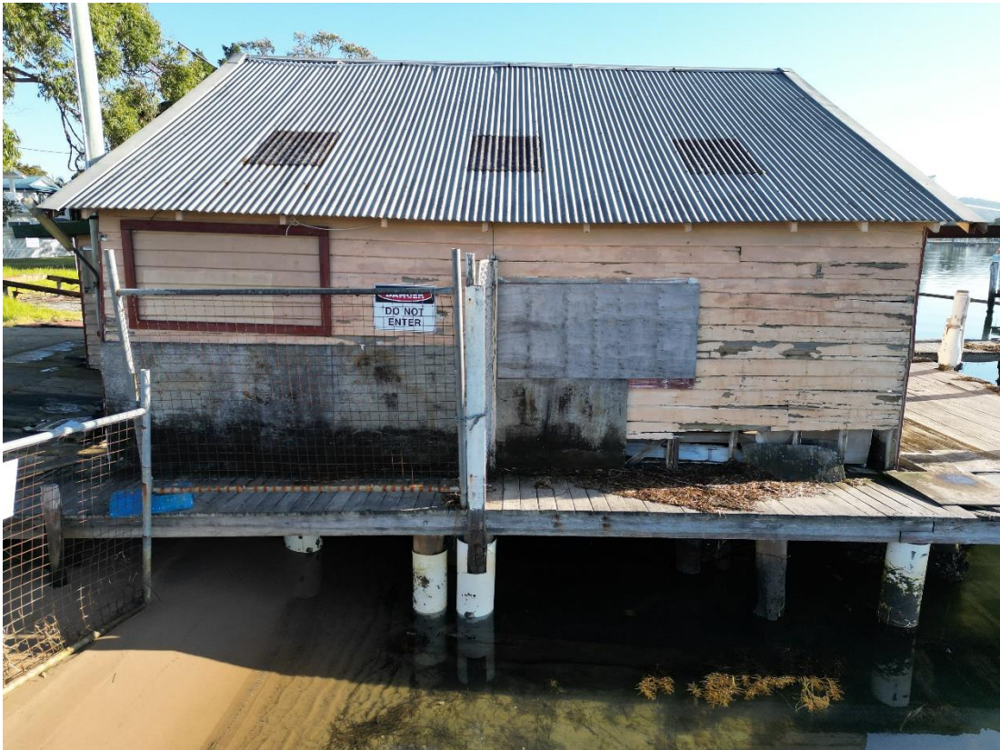
Figure 1.14 – Southern elevation of boat shed with timber walkway to rear landing. Image by Catalyst Consulting.
