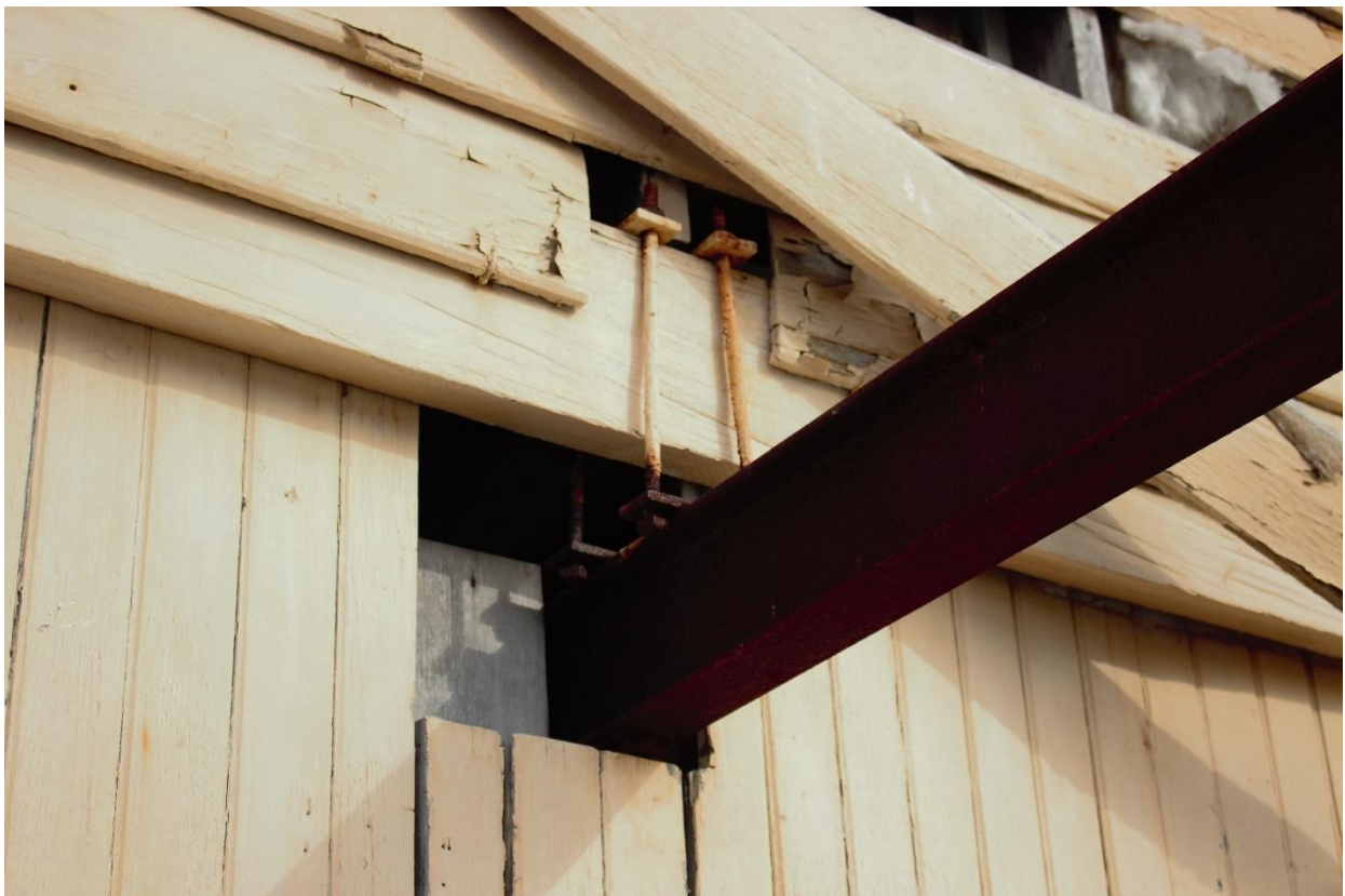
Figure 1.28 – Detail of modification of door for installation of I beam for gantry.
