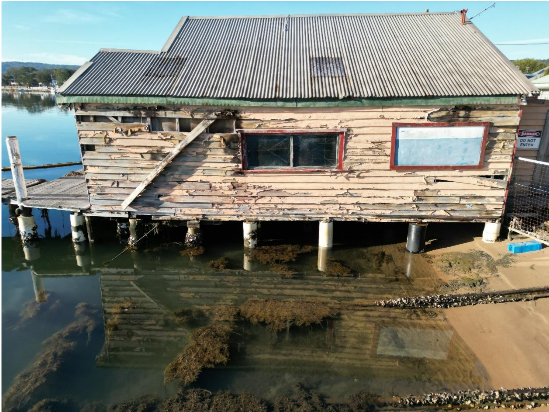
Figure 1.13 – Detail of the northern elevation of the boat shed showing deterioration of timber cladding and slipway rails below HWM. Image by Catalyst Consulting.
