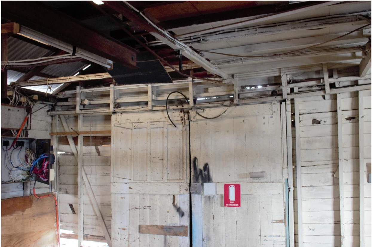
Figure 1.23 – Timber barn style sliding doors – possibly original to 1925. These doors were obscured from view externally.
