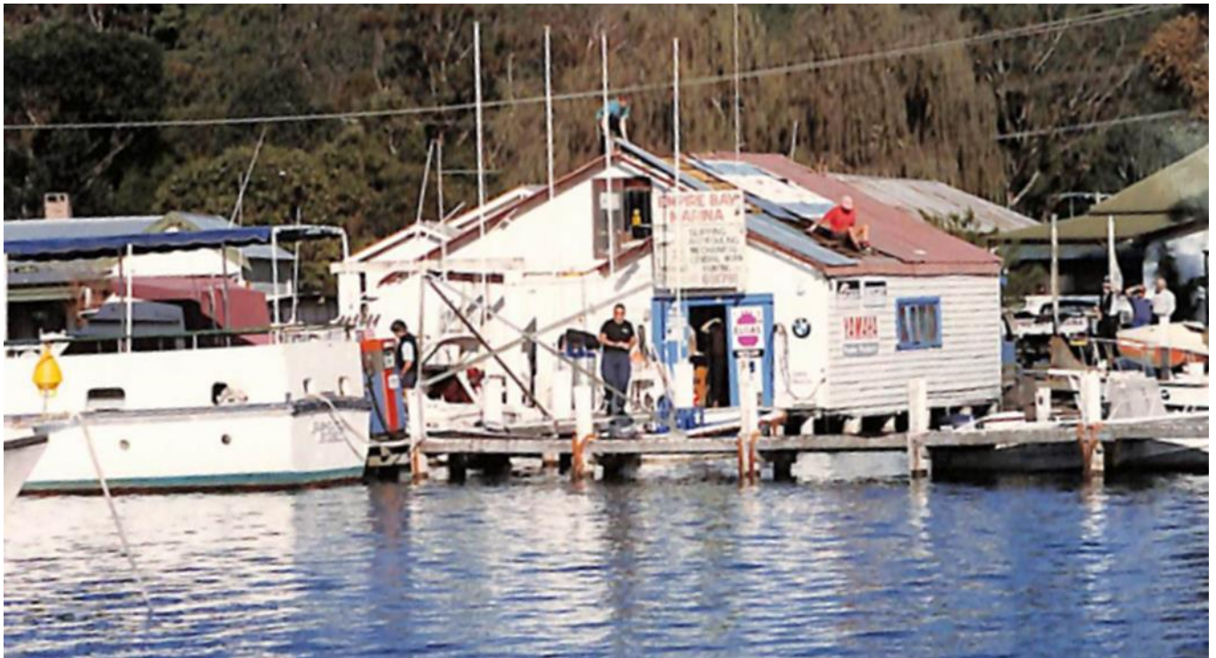
Figure 2.26 – The eastern elevation during the roof replacement. Source: Empire Bay Progress Association.
