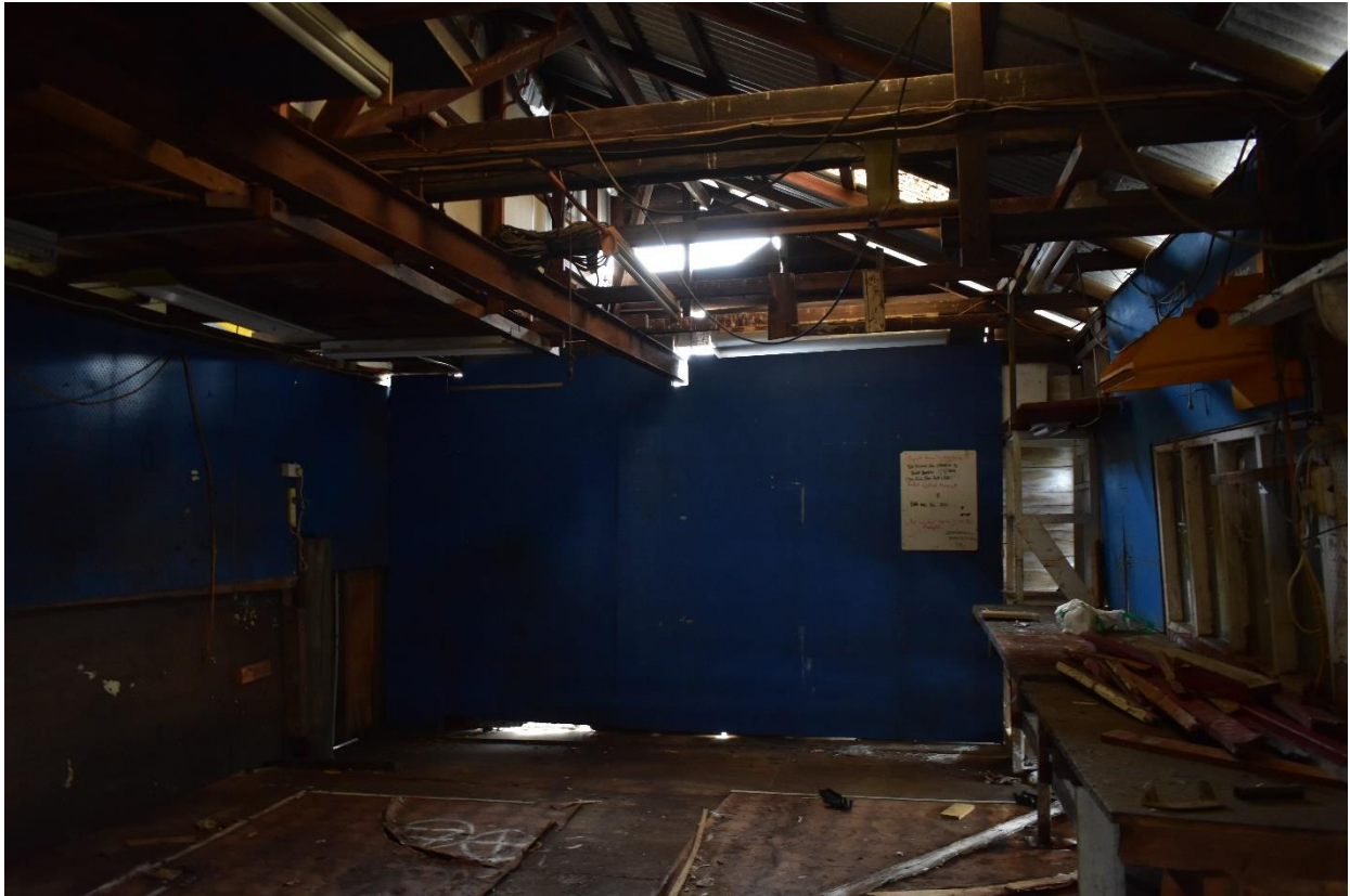
Figure 1.21 – Internal eastern elevation of the boat shed showing roof framing and I beam installed for gantry crane. Sheeting obscured the double doors to the landing.
