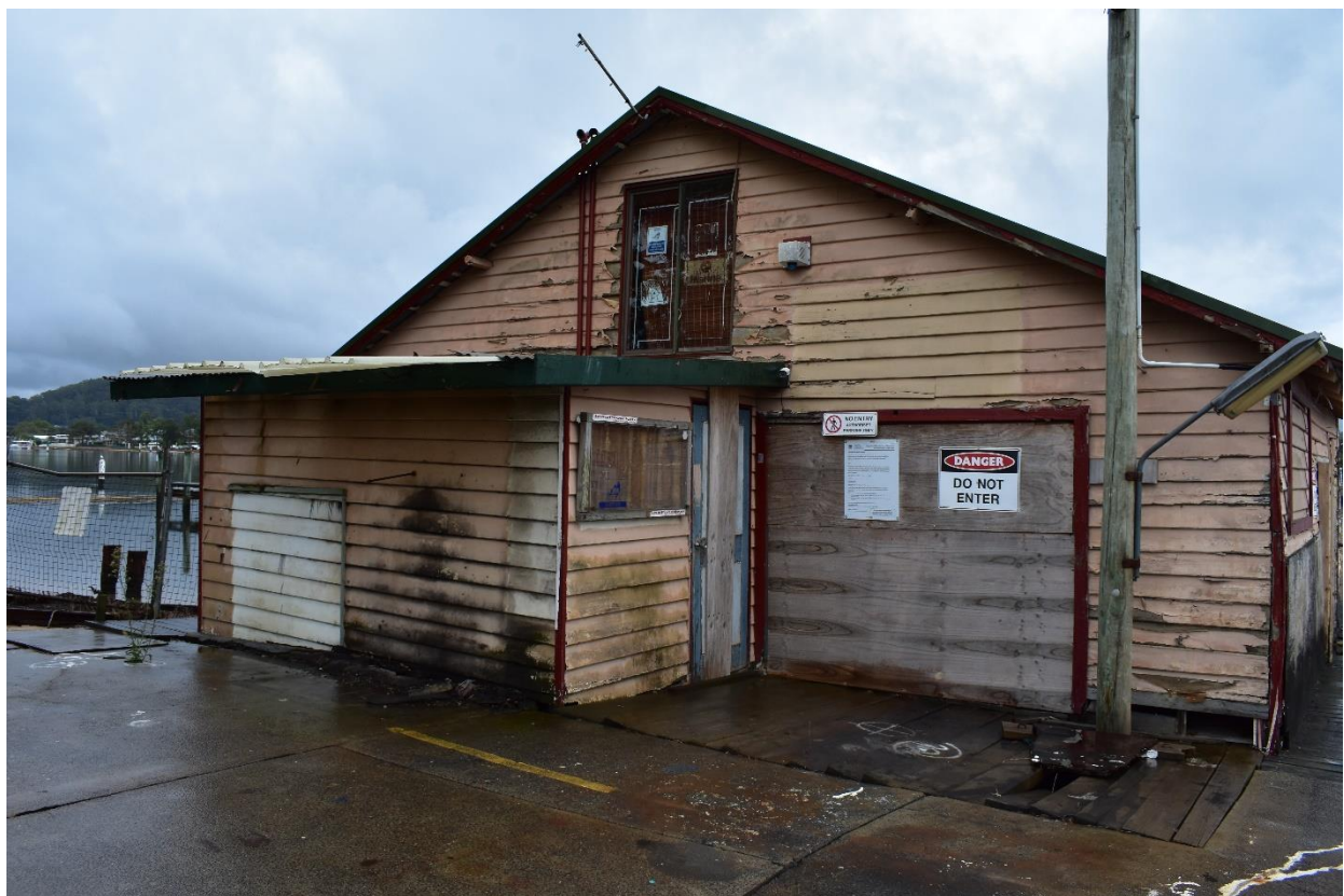
Figure 1.10 – Western elevation of the boat shed showing former doorway, now sealed and obscured, and c1980s addition housing motors for pulley system used to raise boats on slipway.
