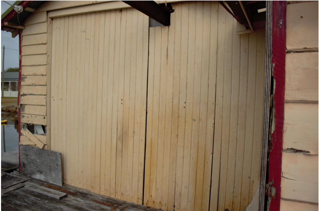
Figure 1.27 – Timber doors on eastern elevation of the boat shed which appear to be original fabric although modified for gantry structure.
